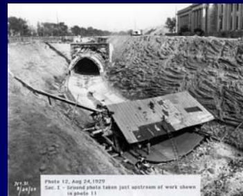
Photo 12, Aug 24, 1929 Fig. 1. Tunnel photo taken just upstream of work shown in photo 11
